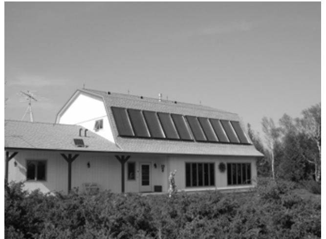
The sun heats this home and its domestic hot water.
